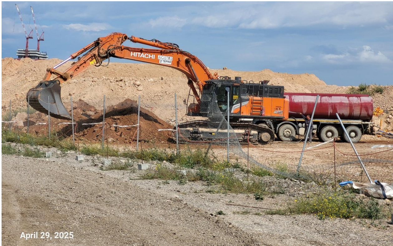
Figure 2.4-4: Wetting of during excavation works as a mitigation measure for dust prevention
