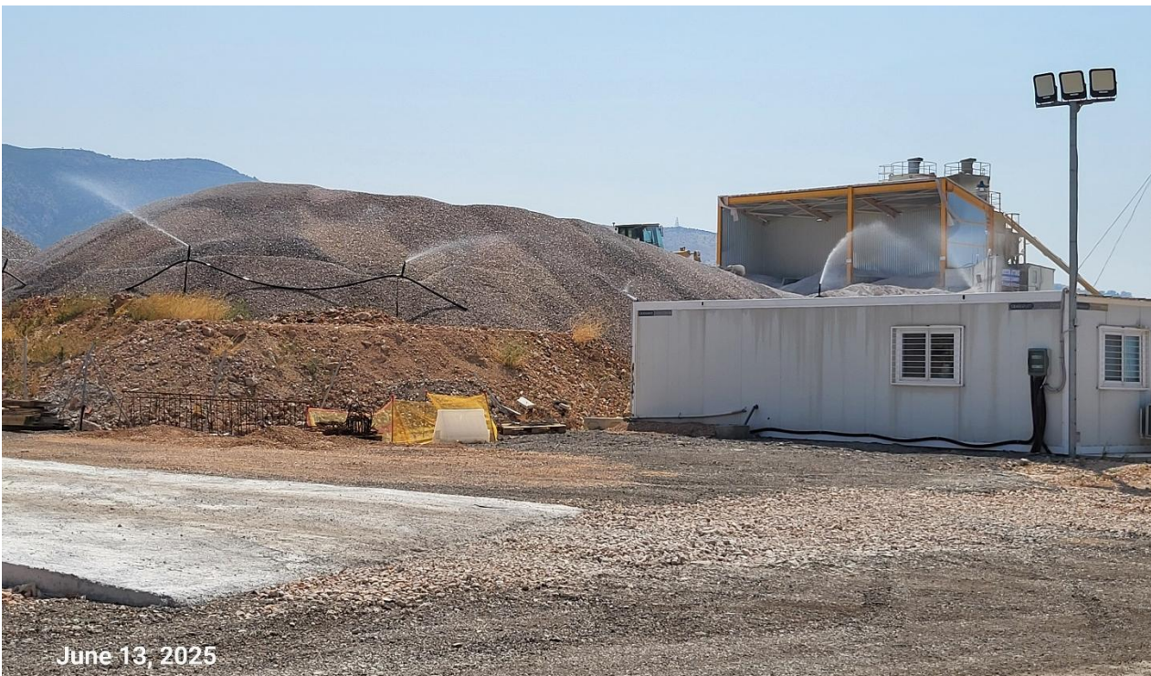
Figure 2.4-5: Wetting of concrete batching plant aggregates stockpile as a mitigation measure for dust prevention
