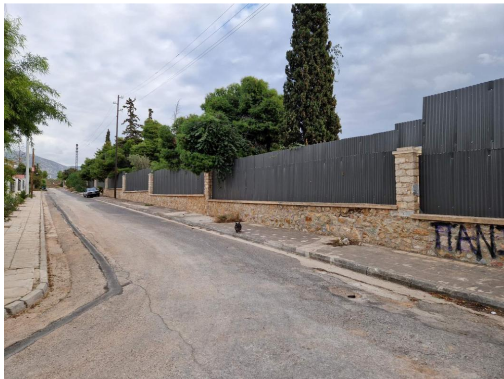
Figure 4.4-3: Noise barriers installed along the fence on Hellinikou and Giota roads
